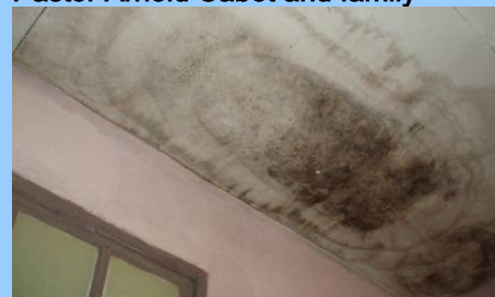
The roof in much need of repair
